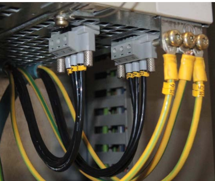
Incorrectly fastened screws pose a serious safety hazard!
